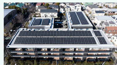
Solar panels installed across the entire rooftop
